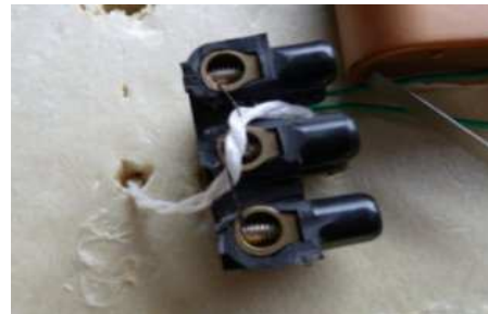
Doc. 8b : Current installation of the resistive wire
